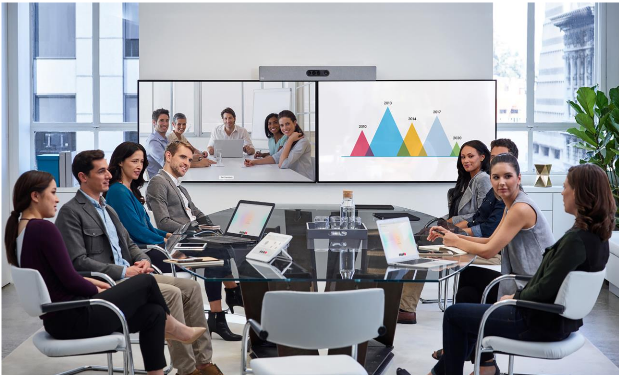
Figure 1. Cisco Spark Room Kit Plus in large conference room
